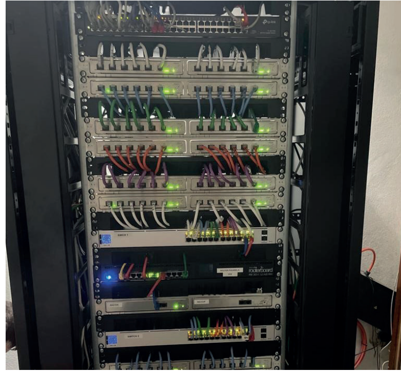
Current innovaphone installation
